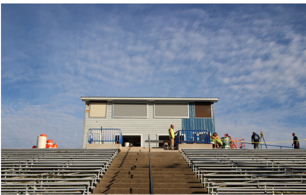
Work is still being done on the pressbox, but it is looking great!
